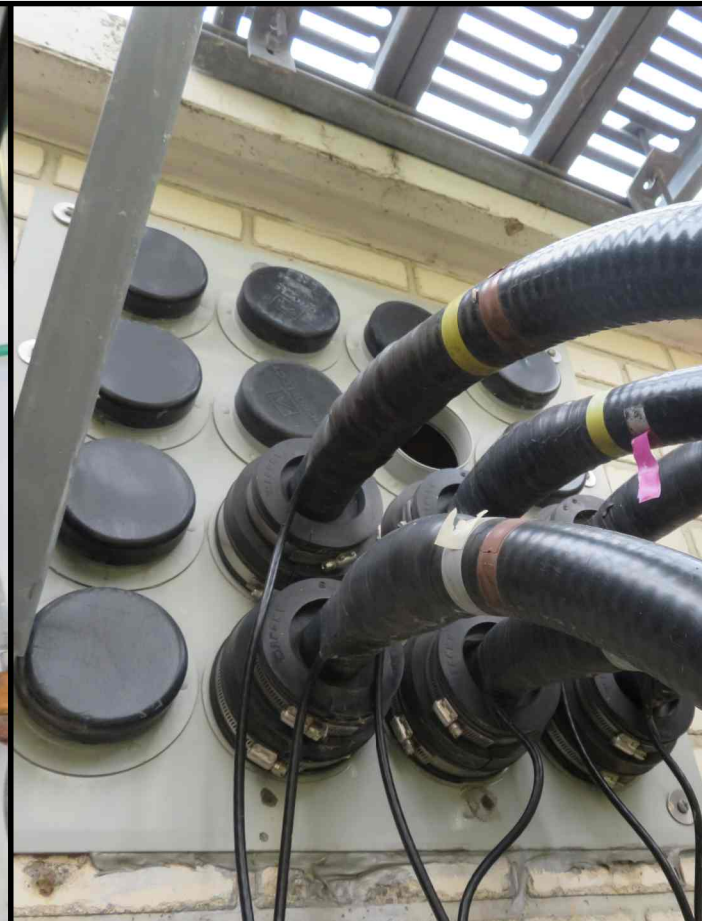
D SHELTER COAX PORT (SHELTER EXTERIOR)
