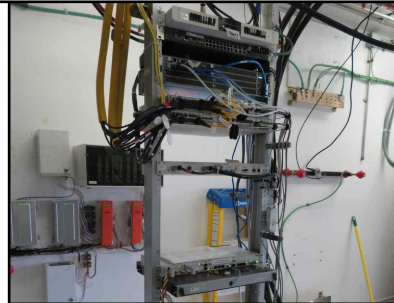
B EXISTING AUX EQUIPMENT RACK
