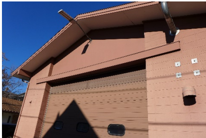
Sagging beam at overhead door
