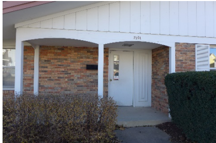
No accessible access to front door
