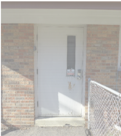
Delamination of back door
