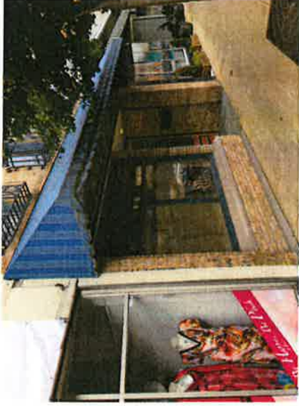
Shows the awning wear and tear
