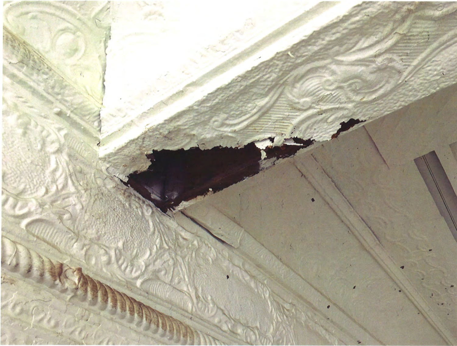
Initial repair of the tin ceiling and walls has included much more than expected patching of rotted tin.
