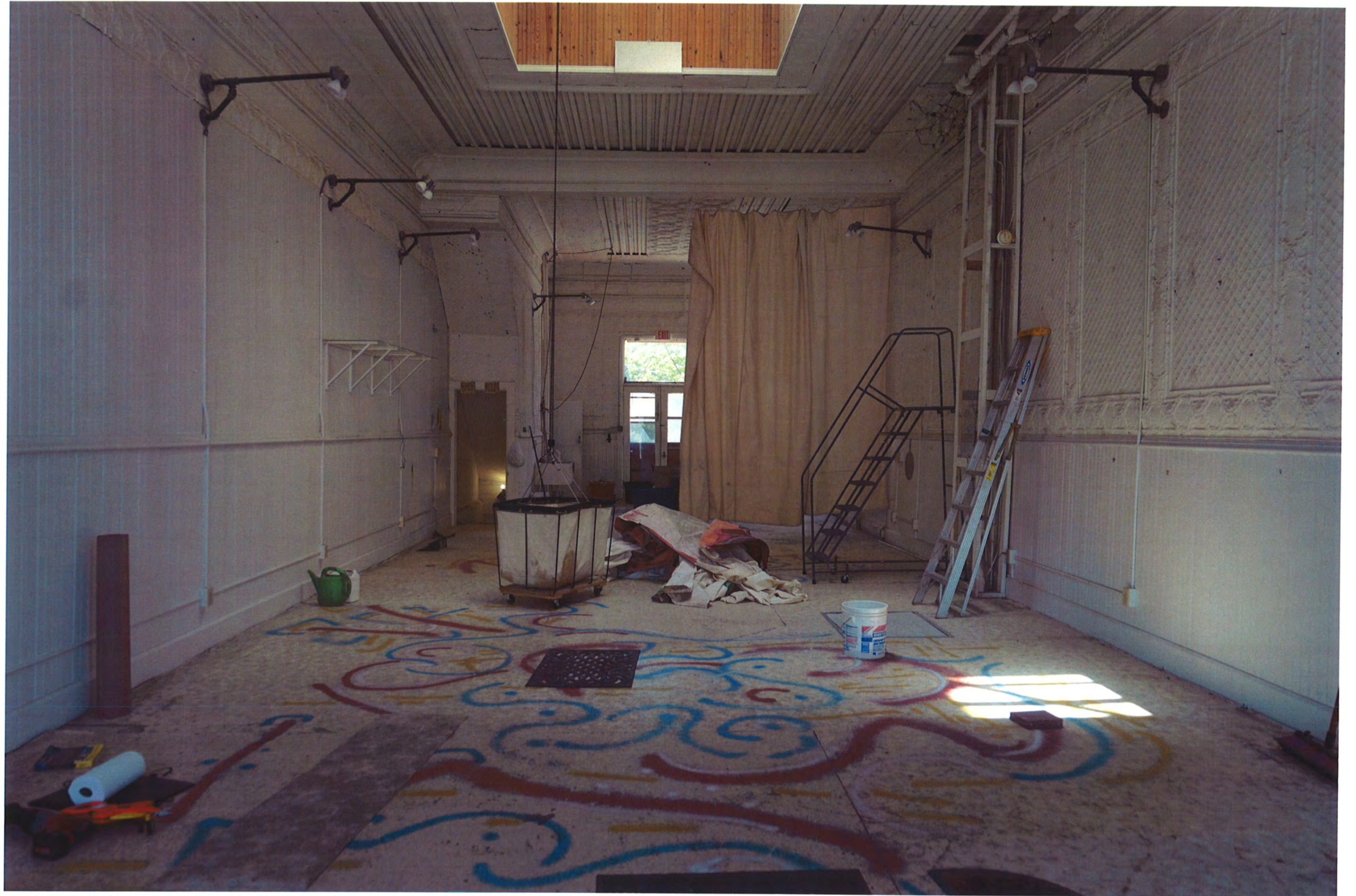
First Floor from Front (Sixth Street) to Back (Seventh Street) Conditions at time of purchase
