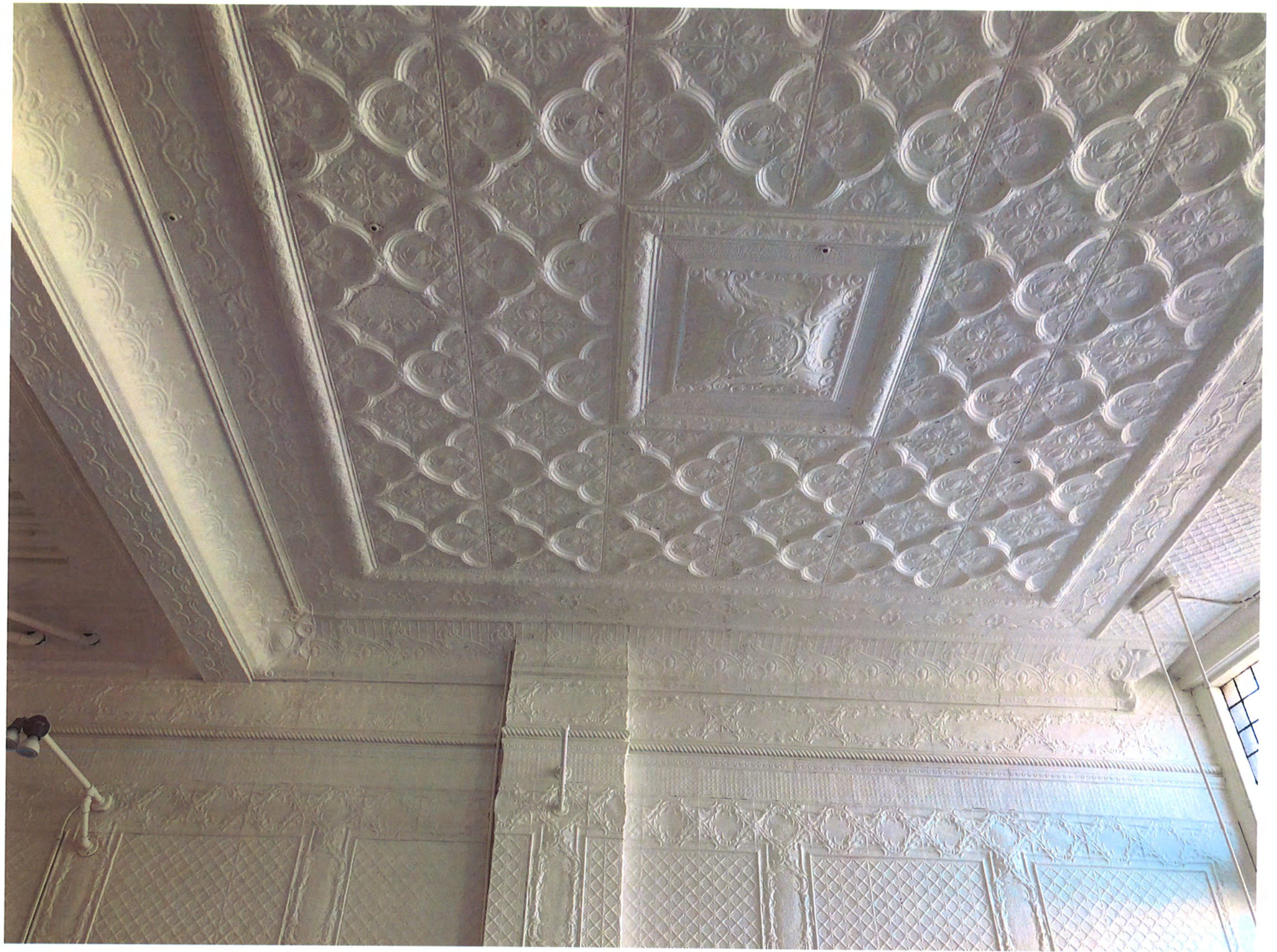
First Floor Ceiling on Sixt Street Conditions now. Tin ceiling and walls repaired and room painted.
