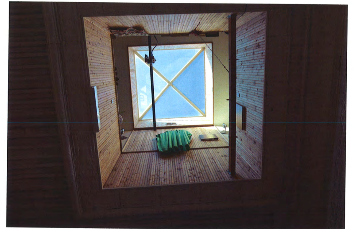
Skylight Shaft Top Right image shows second floor ceiling removed (current conditions.)
