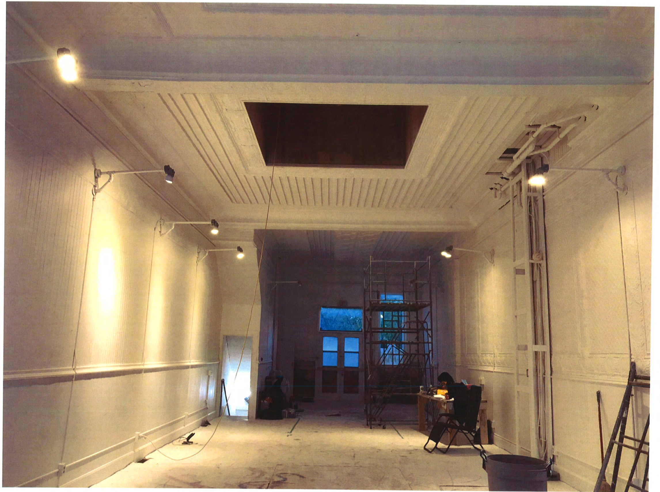
First Floor from Front (Sixth Street) to Back (Seventh Street) Conditions now. Tin ceiling and walls repaired and room painted.
