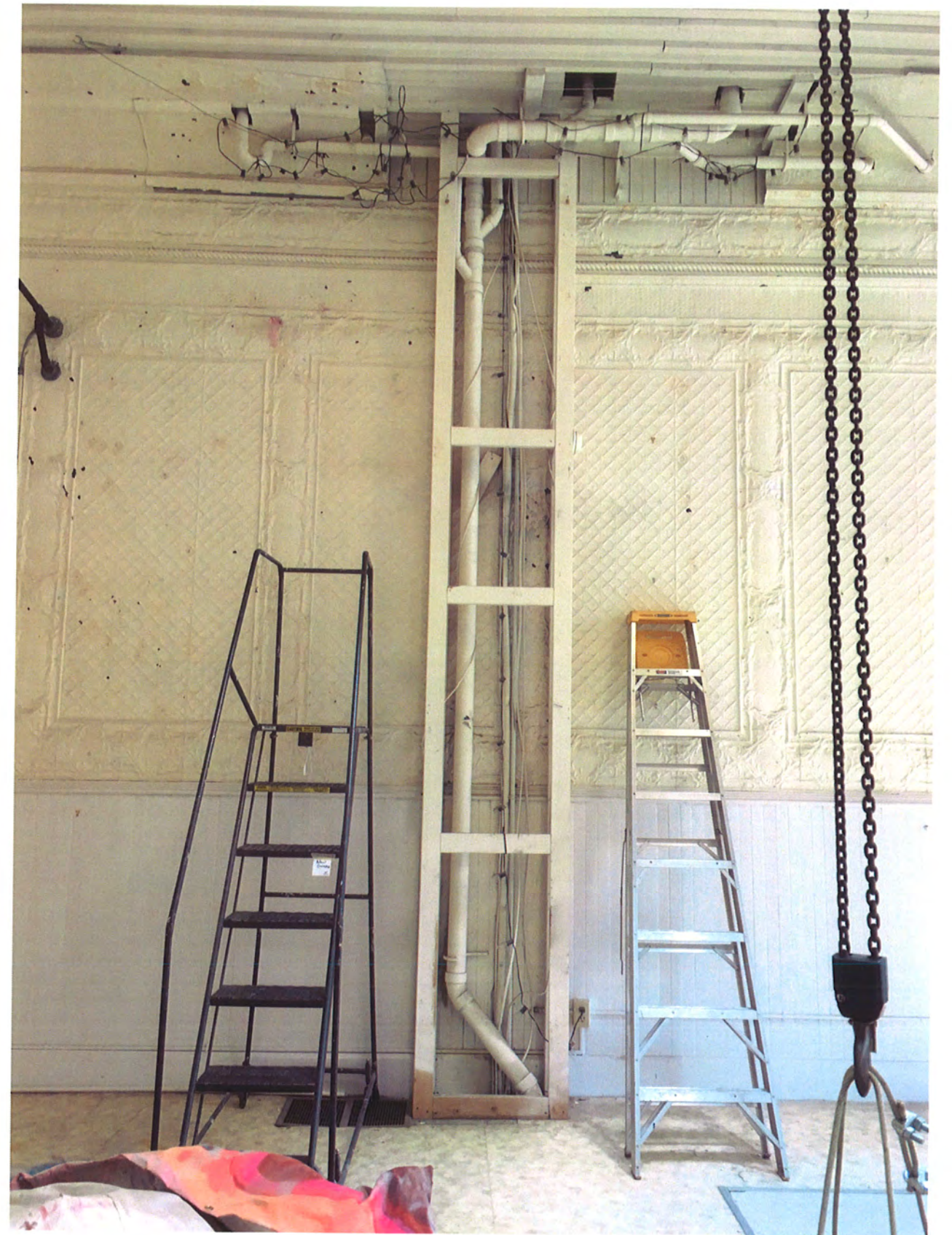
Exposed Plumbing Chase on West Wall to be enclosed, fire stopped and used as destratification ductwork.
