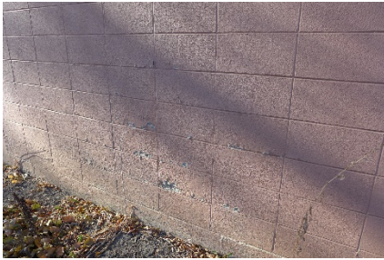
Spalling CMU walls at App. Bay
