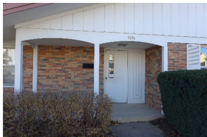
No accessible access to front door
