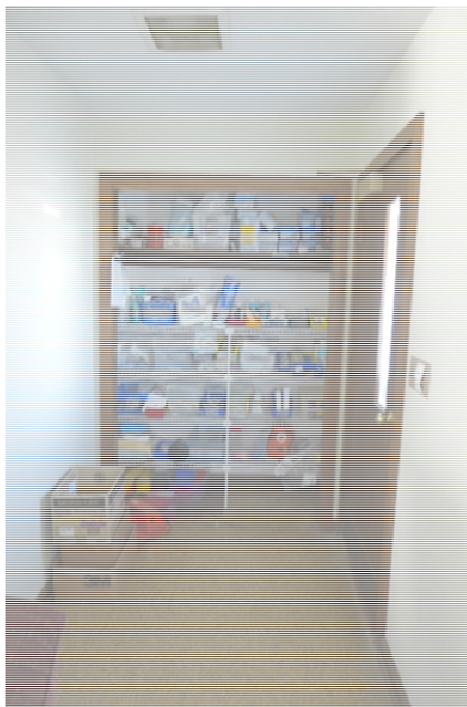
Lack of security for EMS supplies
