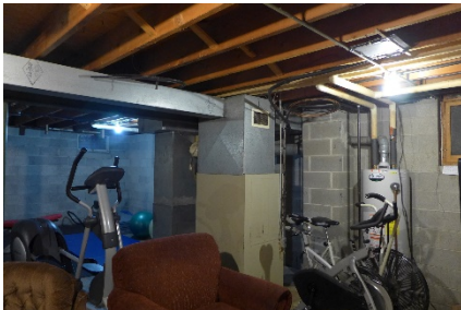
Furnace and water heater
