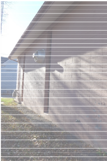
Spalling CMU walls at App. Bay
