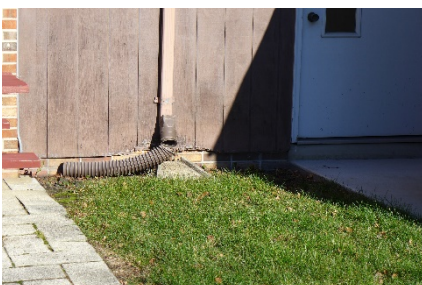
Broken downspout allowing water to collect near foundation wall.
