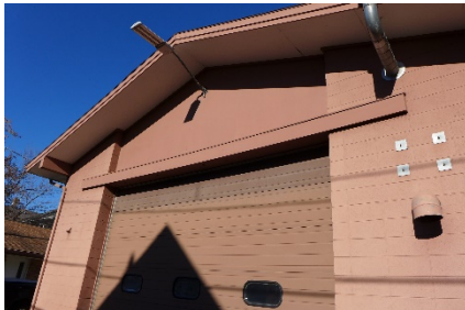
Sagging beam at overhead door
