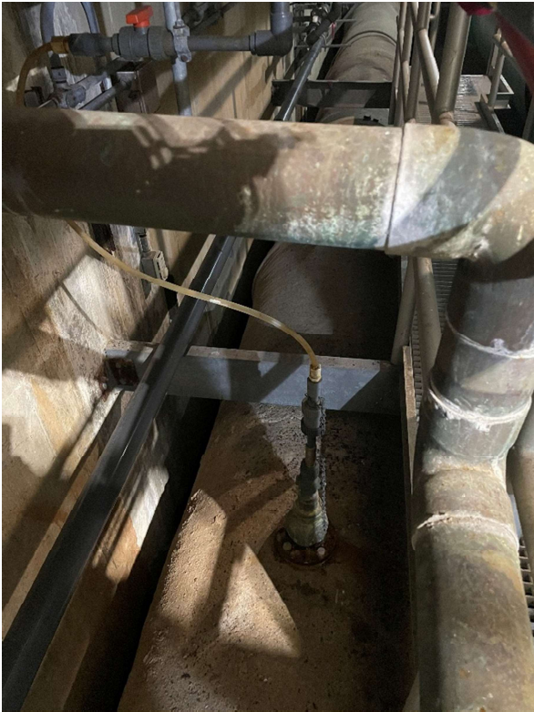
Figure 2 – Existing Filter Aid Polymer (FAP) Injection Tap on the Raw Water Line.
