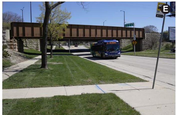
MCTS Route 51 bus passes under the UP bridge over Oklahoma Ave. This single-track bridge dates to construction of the I-794 project.
